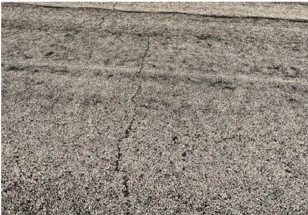
Another area of lateral cracking
