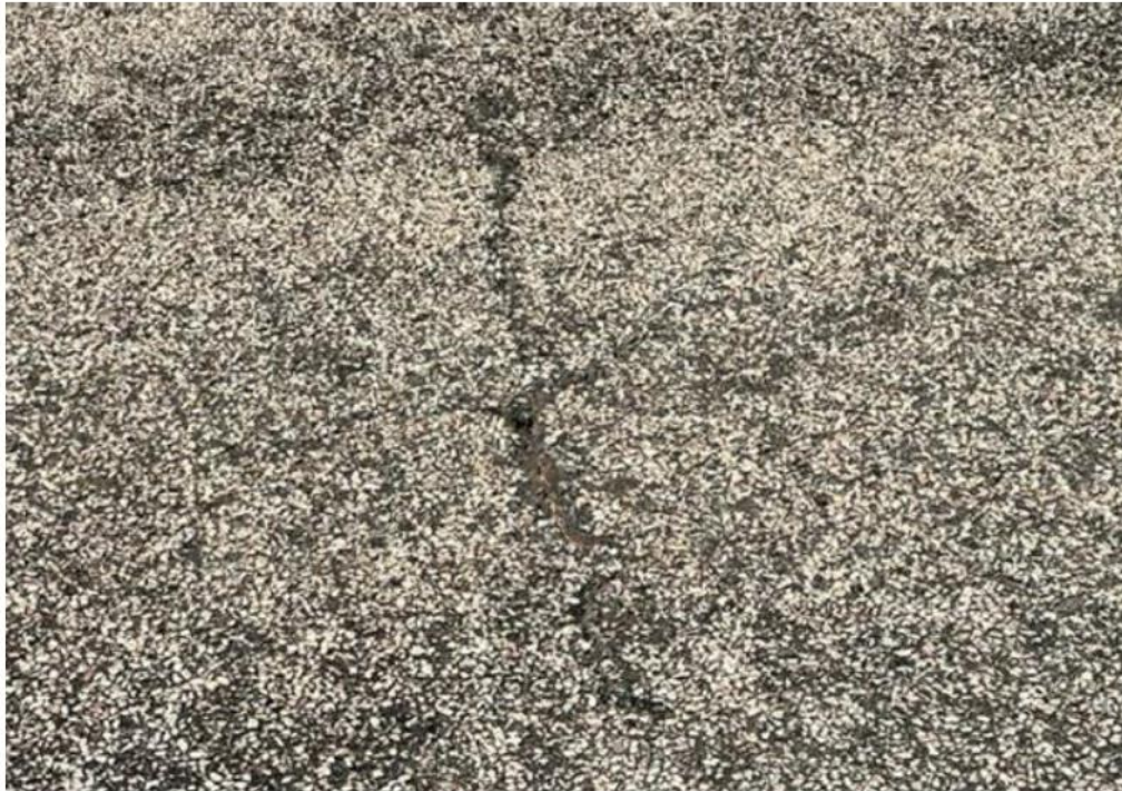
Some open cracking towards the east end, south side
