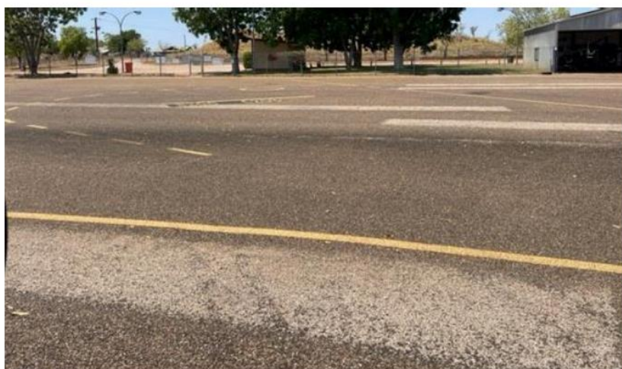
Apron showing stone stripping
