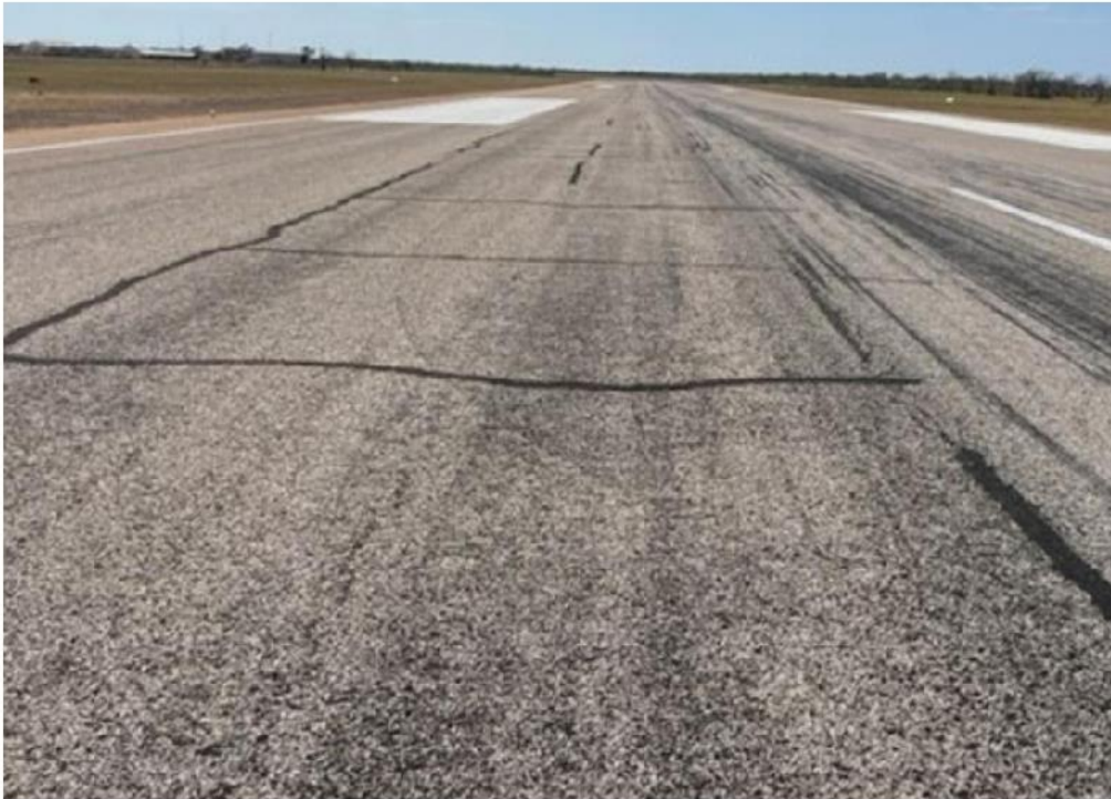
Areas where ground staff have done an excellent job in crack patching
