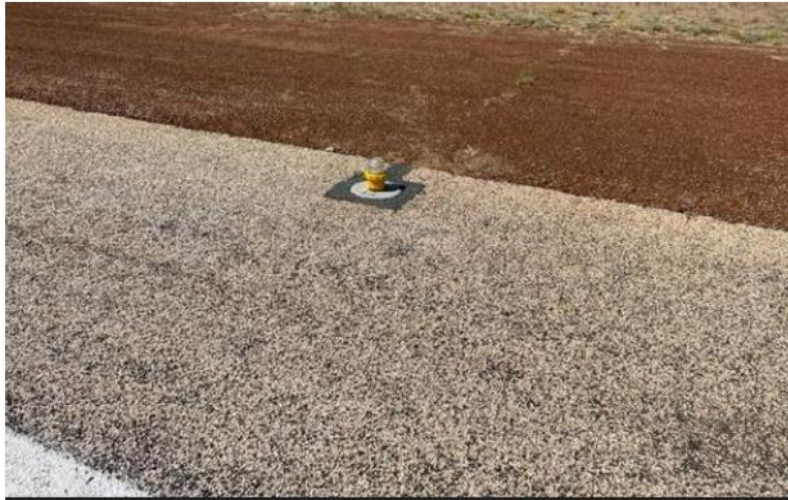
Low Intensity Runway Lighting in situ
