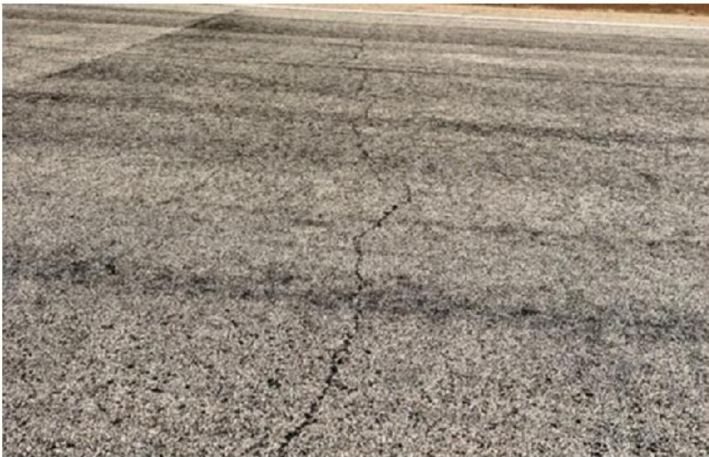
Cracking occurring in a lateral direction in some areas.
