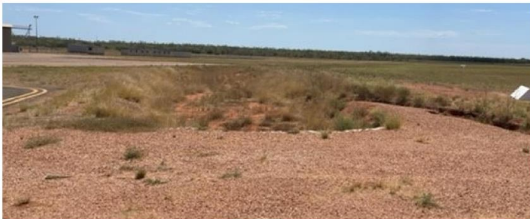
Drain requiring regrading
