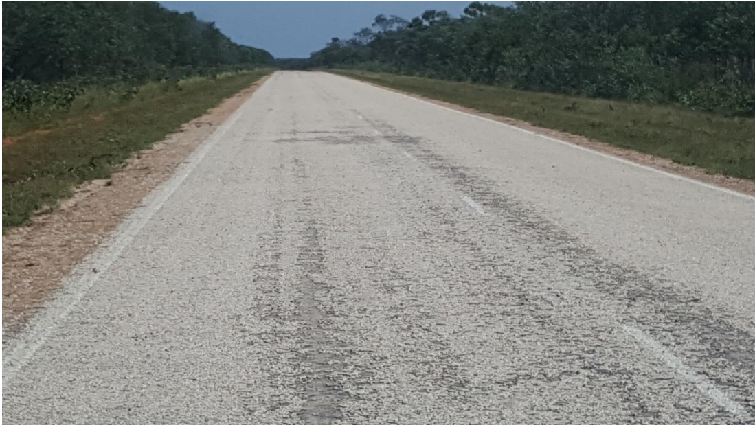
Ravelling (fretting), Curtin Access Rd – Condition 5, Very Poor
