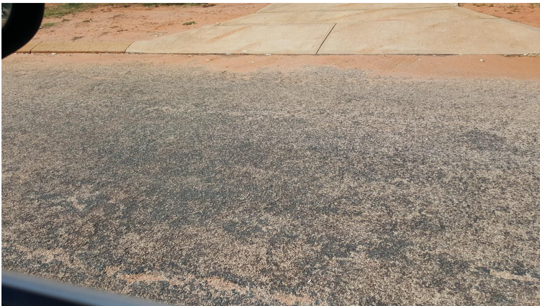
Polishing, Short St – Condition 5, Very Poor
