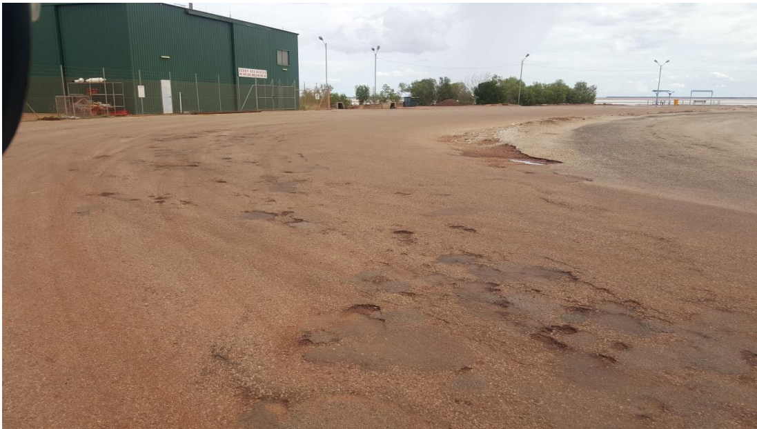
Potholing, Jetty Boat Ramp Access Road – Condition 5, Very Poor
