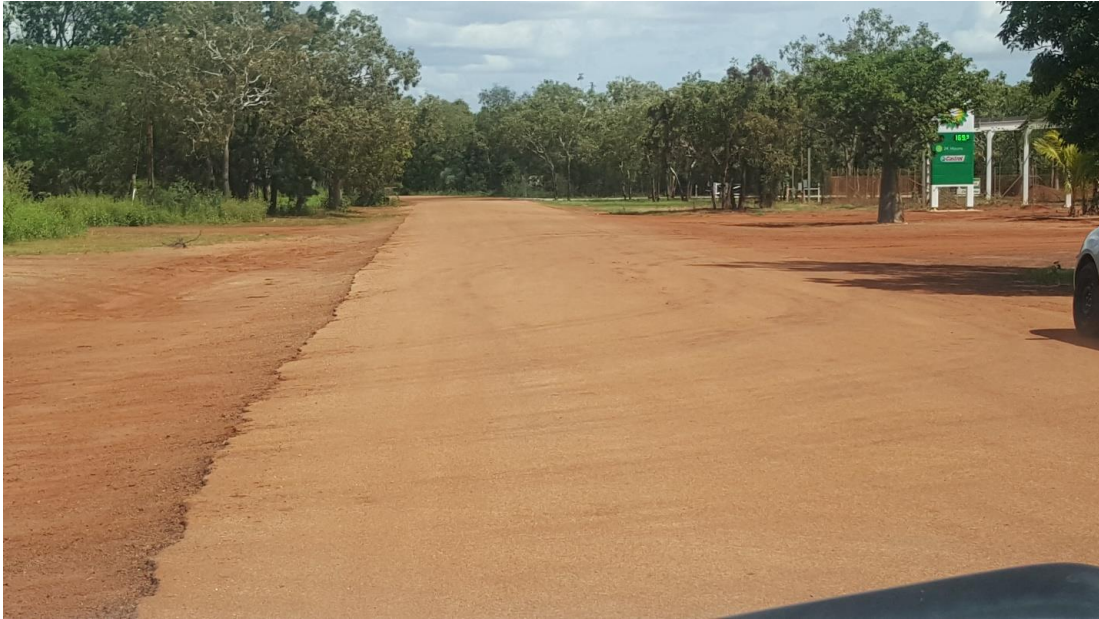
Edge Drop Off, Rodgers St – Condition 4, Poor
