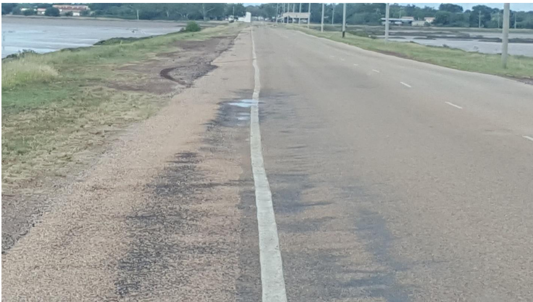
Deformation (rutting), Jetty Rd – Condition 4, Poor
