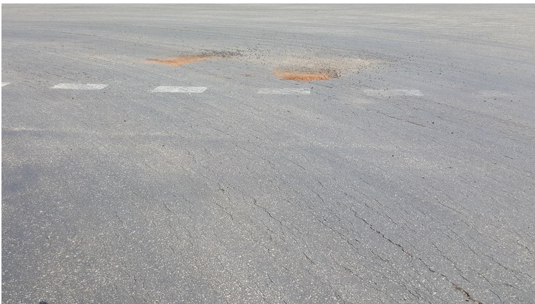
Deformation (shoving), Jetty Access Road – Condition 4, Poor
