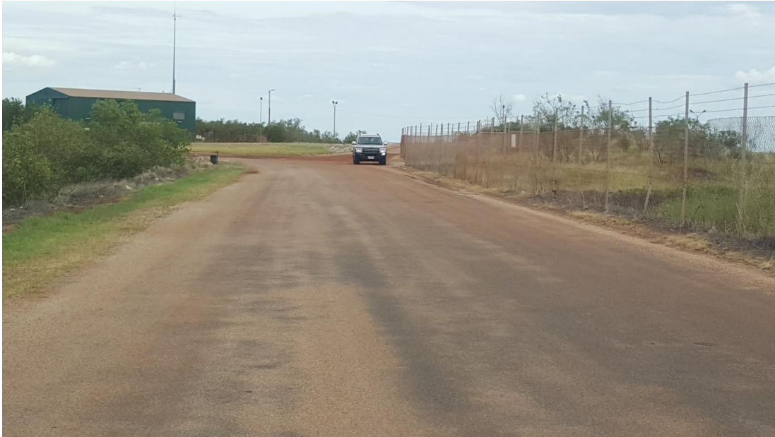
Flushing (bleeding), Jetty Boat Ramp Access Road – Condition 5, Very Poor
