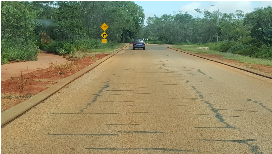
Block Cracking, Fitzroy St – Condition 3, Fair
