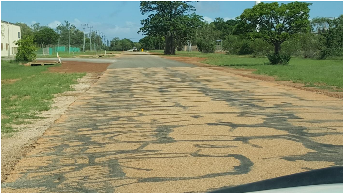
Transverse Cracking, Wodehouse St – Condition 5, Very Poor
