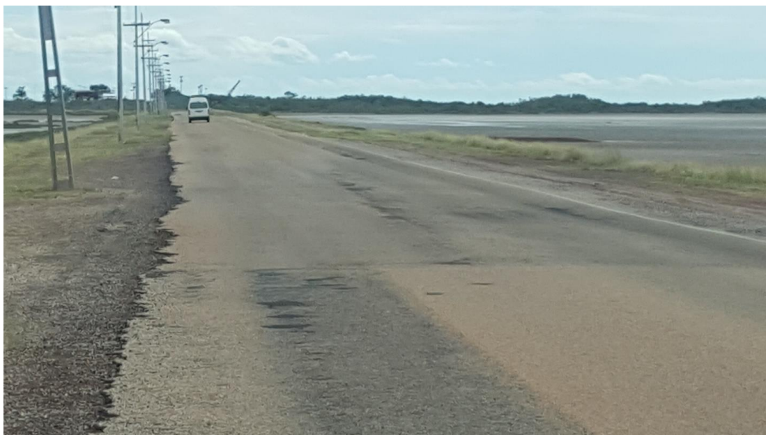
Edge Break, Jetty Rd – Condition 4, Poor
