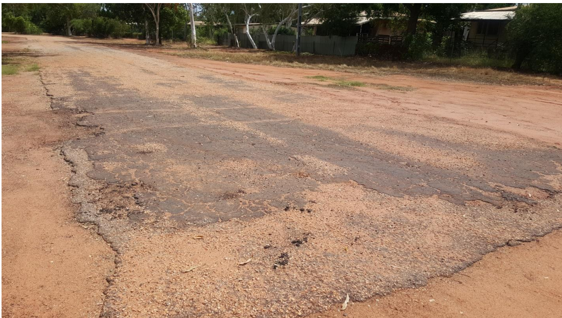
Stripping, Rowell Crt – Condition 5, Very Poor
