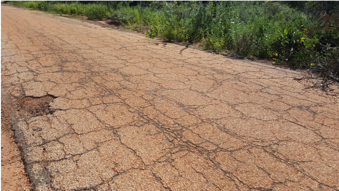
Crocodile Cracking, Granville St – Condition 5, Very Poor
