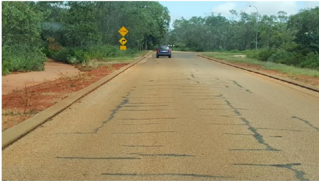
Block Cracking, Fitzroy St – Condition 3, Fair
