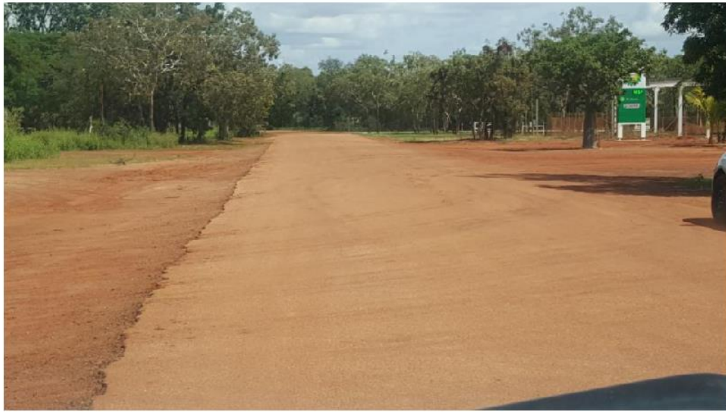
Edge Drop Off, Rodgers St – Condition 4, Poor
