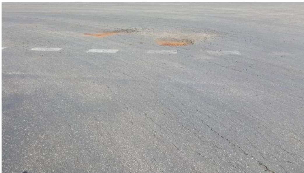
Deformation (shoving), Jetty Access Road – Condition 4, Poor
