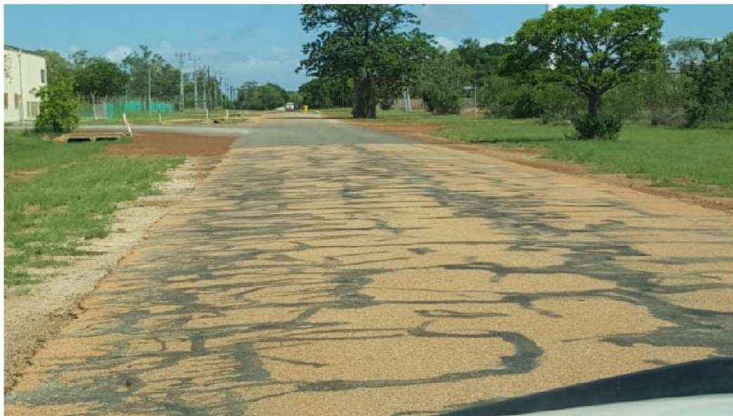
Transverse Cracking, Wodehouse St – Condition 5, Very Poor
