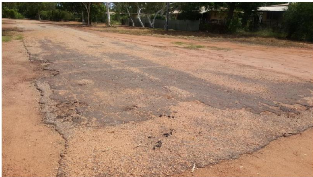
Stripping, Rowell Crt – Condition 5, Very Poor
