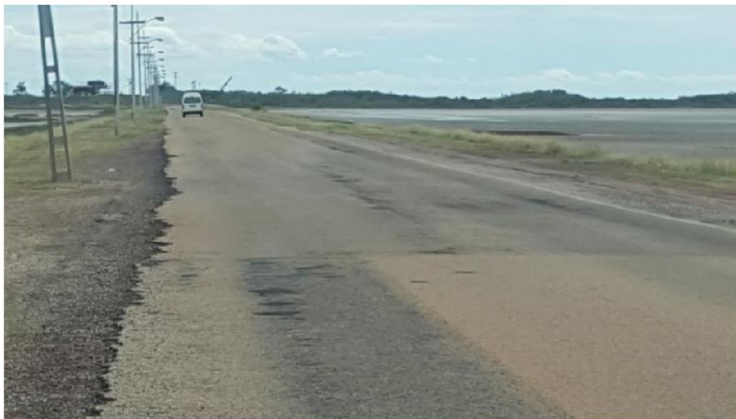
Edge Break, Jetty Rd – Condition 4, Poor
