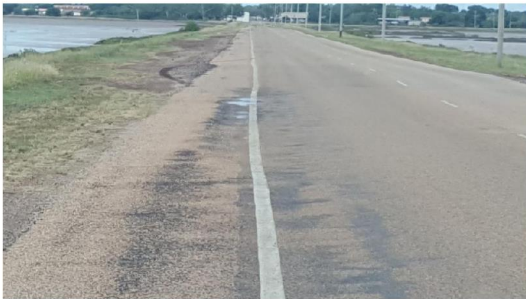
Deformation (rutting), Jetty Rd – Condition 4, Poor
