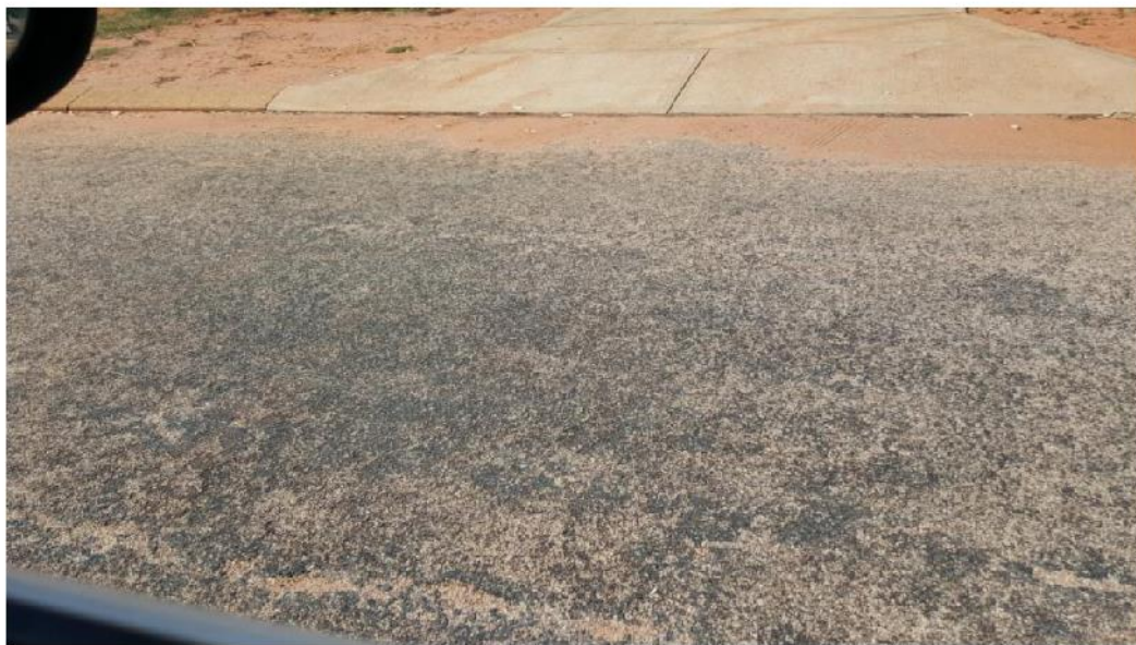
Polishing, Short St – Condition 5, Very Poor
