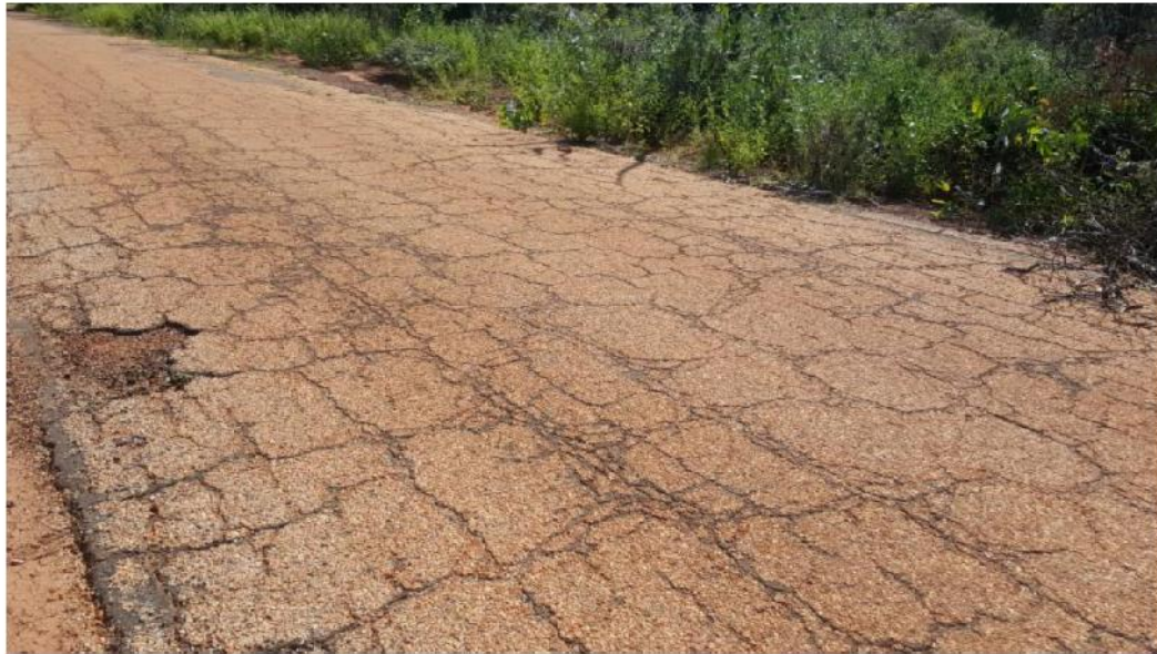
Crocodile Cracking, Granville St – Condition 5, Very Poor
