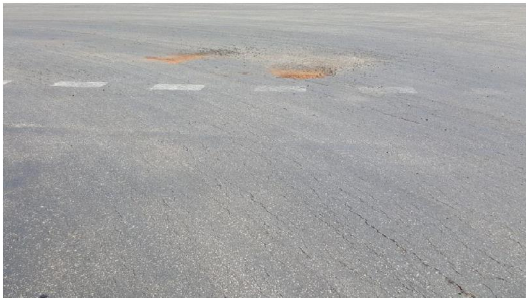
Deformation (shoving), Jetty Access Road – Condition 4, Poor
