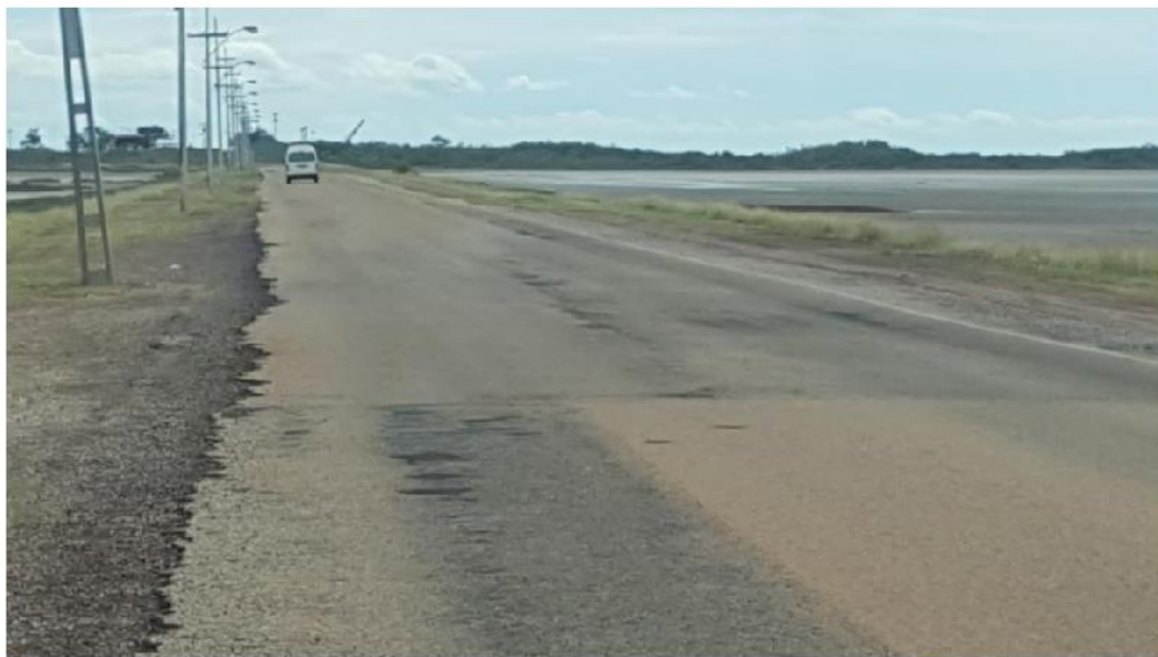
Edge Break, Jetty Rd – Condition 4, Poor
