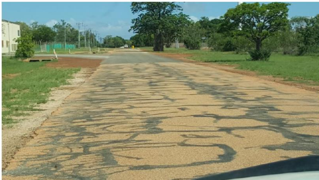
Transverse Cracking, Wodehouse St – Condition 5, Very Poor
