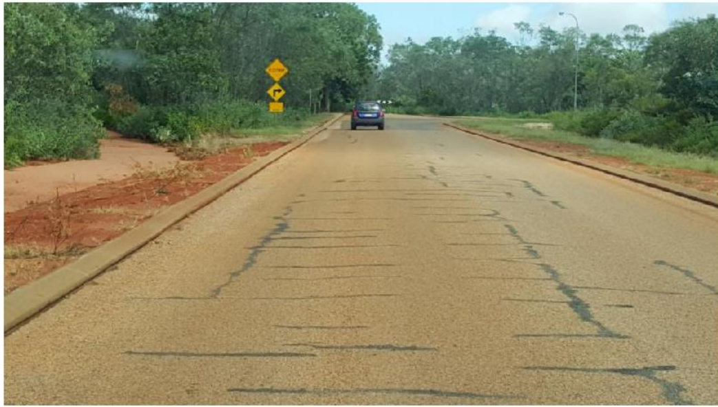
Block Cracking, Fitzroy St – Condition 3, Fair
