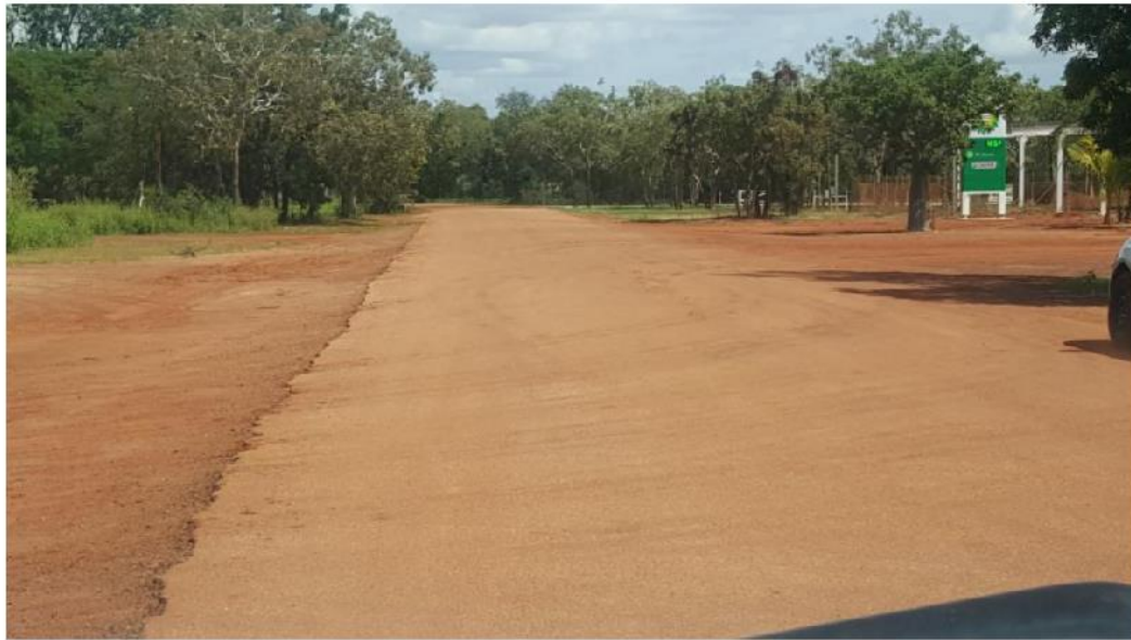
Edge Drop Off, Rodgers St – Condition 4, Poor
