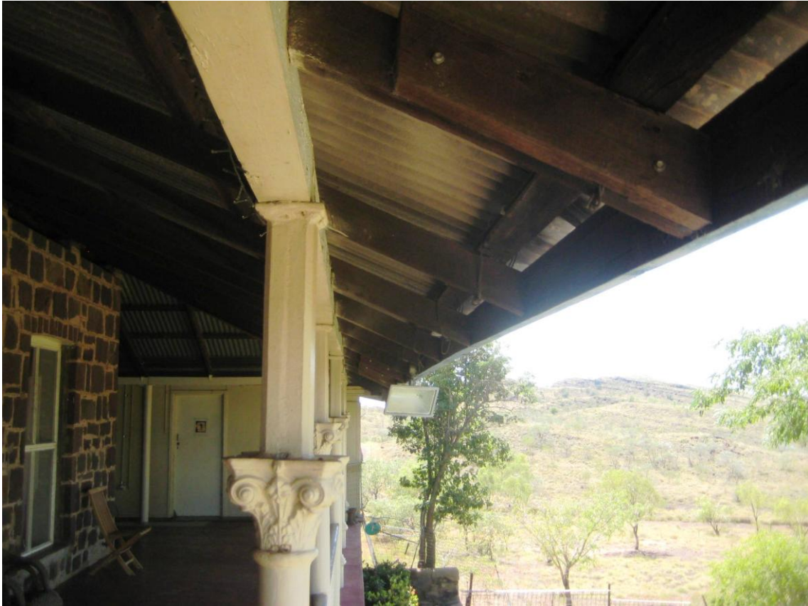
▲ P5 Eastern side verandah of Liveringa Homestead showing column, beam and rafter detailing (JTA 27 April 2016)
