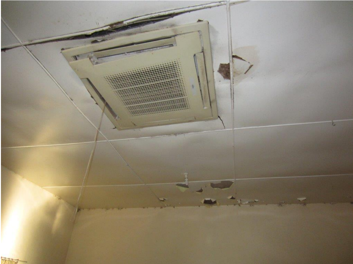
▲ P7 Damaged battened masonite ceilings in the three central rooms of Liveringa Homestead (Brett Blanchett March 2015)
