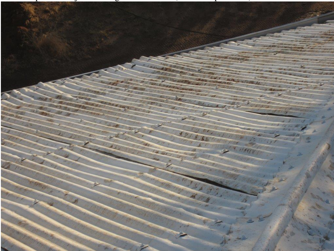
▲ P4 Illustration of Liveringa Homestead roof corrosion (Brett Blanchett March 2015)
