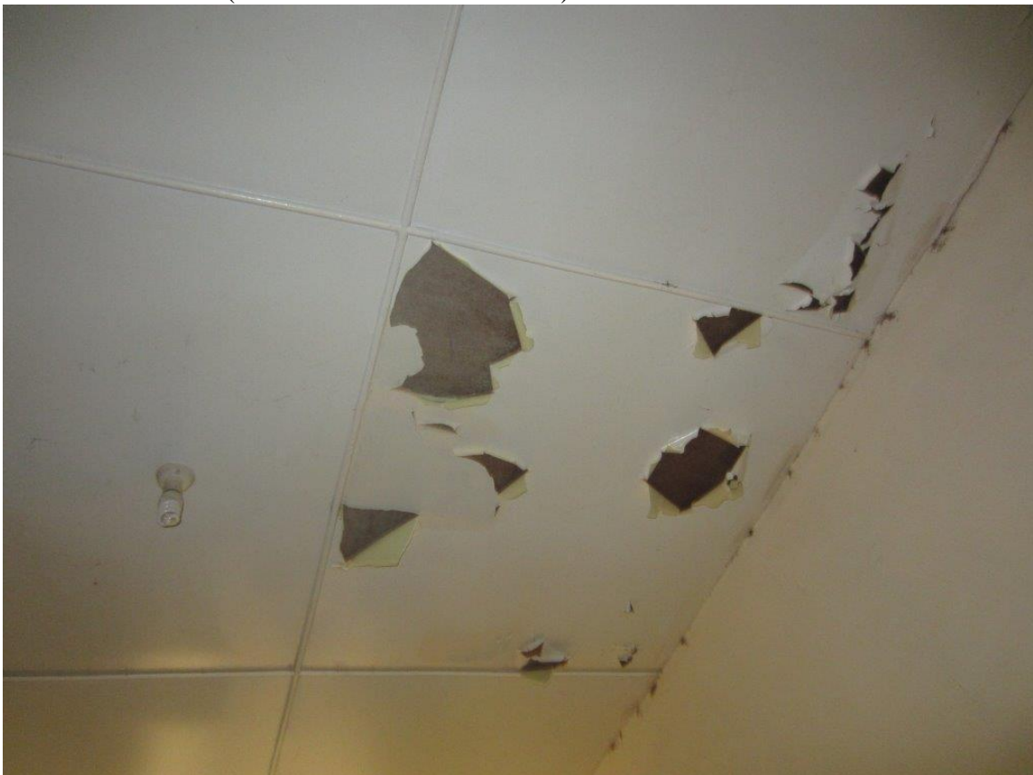
▲ P8 Damaged battened masonite ceilings in the three central rooms of Liveringa Homestead (Brett Blanchett March 2015)
