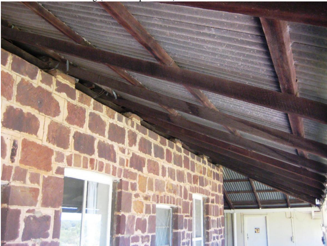
▲ P6 Eastern side verandah of Liveringa Homestead showing wall plate, rafter and purlin detailing (JTA 27 April 2016)
