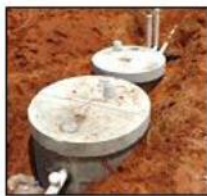
Unsealed or damaged septic tanks or open leach drains
