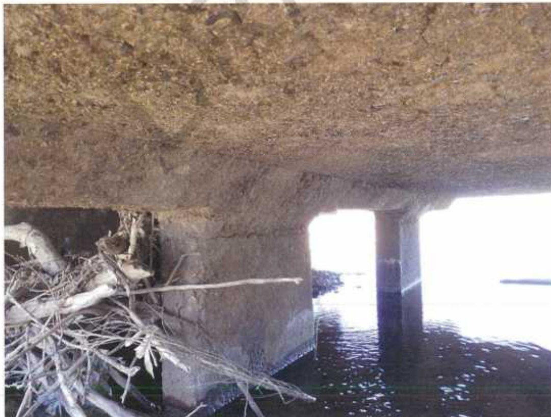
Photo No. 30: LHS at pier 30 (A1 side), legs and top deck to span 30. (Taken: 20-Jun-2016)
