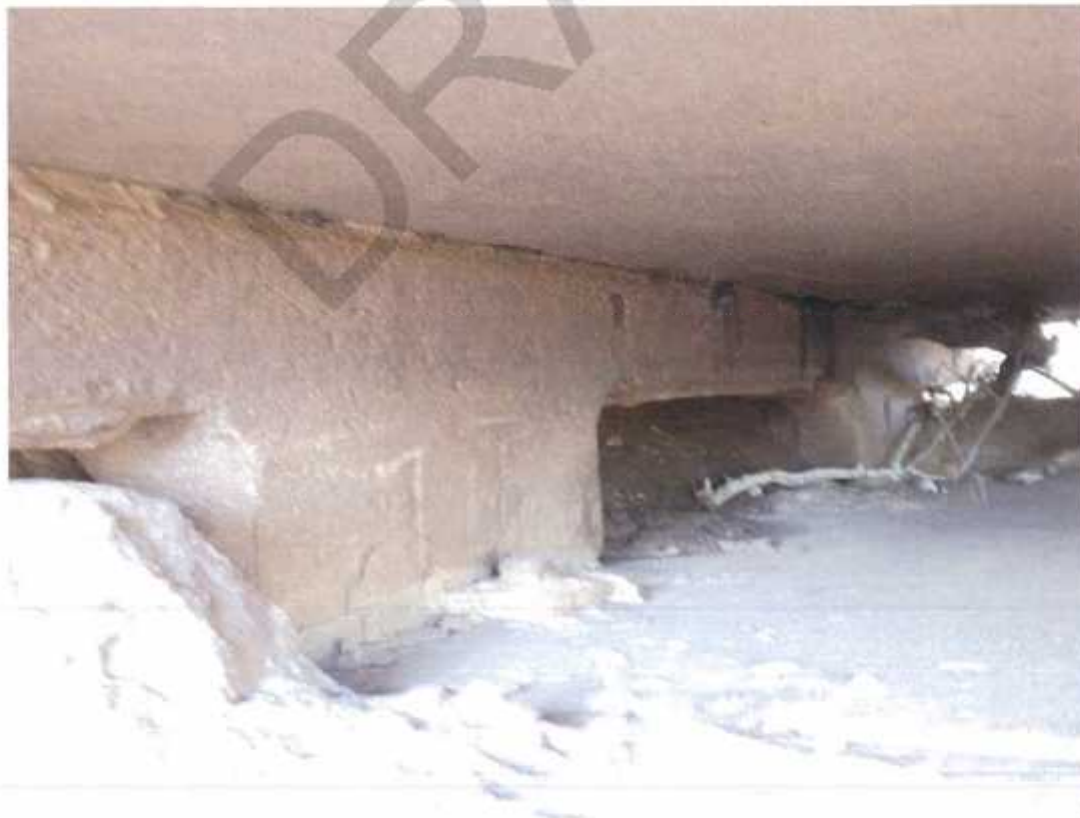
Photo No. 50: RHS, A2 legs spalled, typical. (Taken: 20-Jun-2016)
