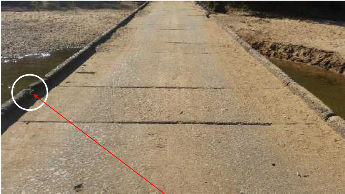
140312 – Reinforcing steel exposed
