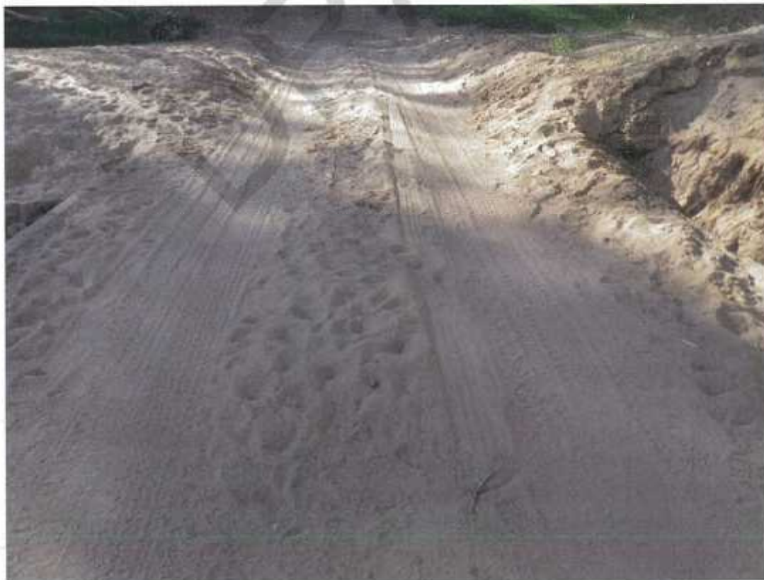
Photo No. 14: Build up of sand covering the first four spans (Taken: 20-Jun-2016)
