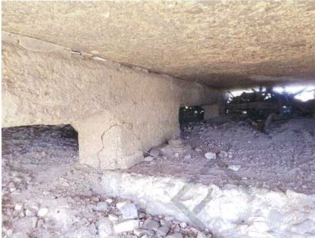
Photo No. 47: RHS at pier 8, A1 legs spalled. (Taken: 20-Jun-2016)
