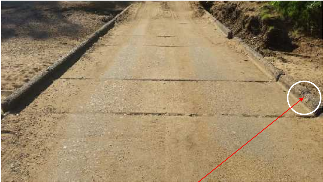
140336 – Reinforcing steel exposed
