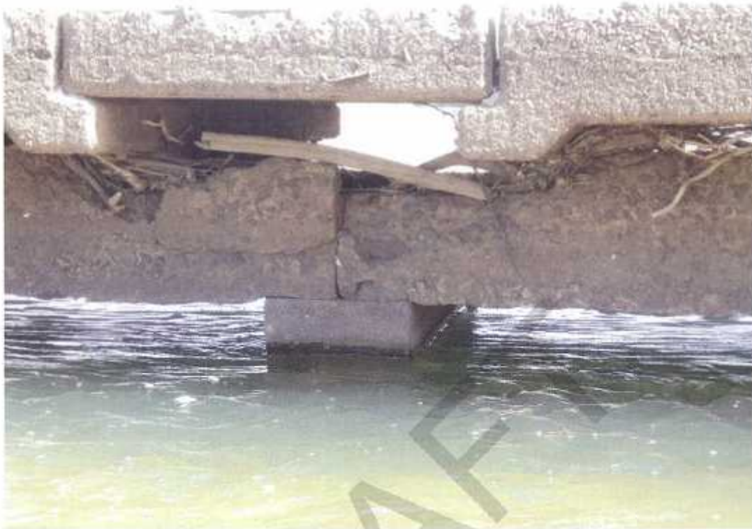
Photo No. 21: LHS span 10, cracking/ spalling tc kerb edge. (Taken: 20-Jun-2016)
