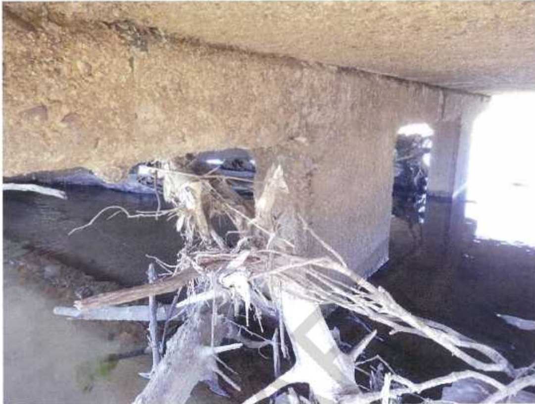
Photo No. 29: LHS at pier 24, legs to top deck. Original deck under water. (Taken: 20-Jun-2016)
