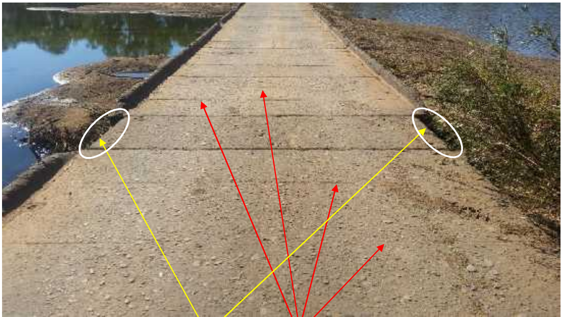
Kerbs missing - 135838 – Lateral grooves
