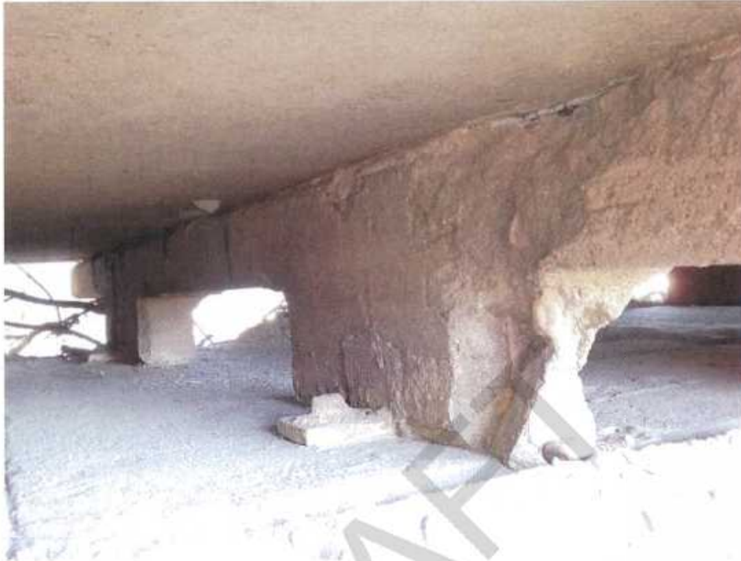
Photo No. 49: RHS, A2 legs spalled, typical. (Taken: 20-Jun-2016)
