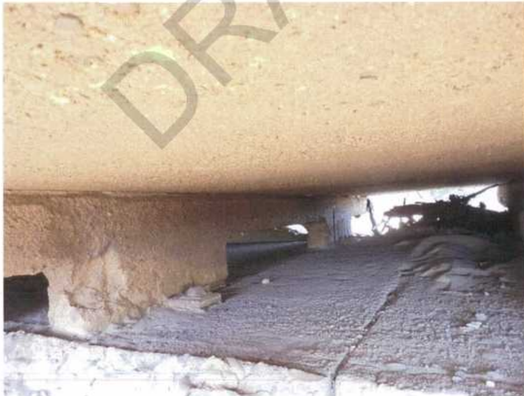
Photo No. 48: RHS at pier 8, A1 legs spalled. (Taken: 20-Jun-2016)
