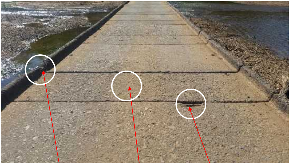
Spalling of kerb – 140154 – Longitudinal crack & reinforcing steel exposed
