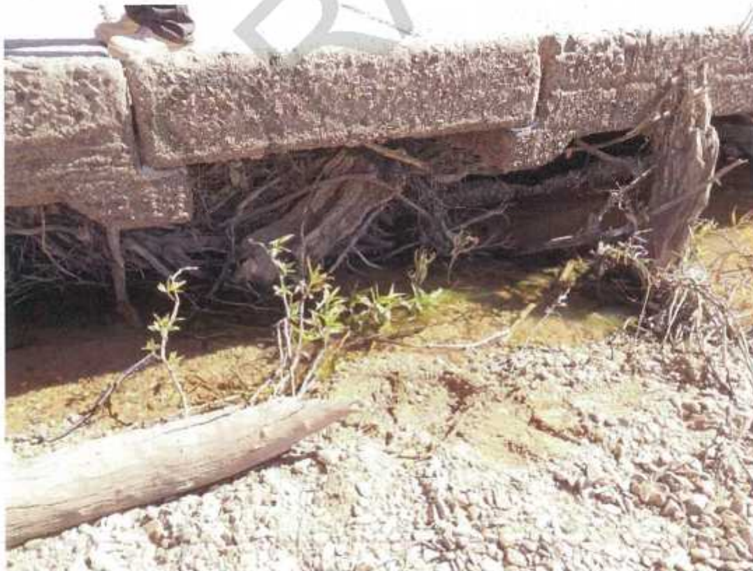
Photo No. 28: LHS at pier 23, flood debris. (Taken: 20-Jun-2016)
