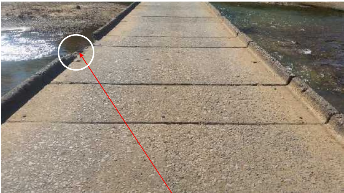
140217 – Part kerb missing
