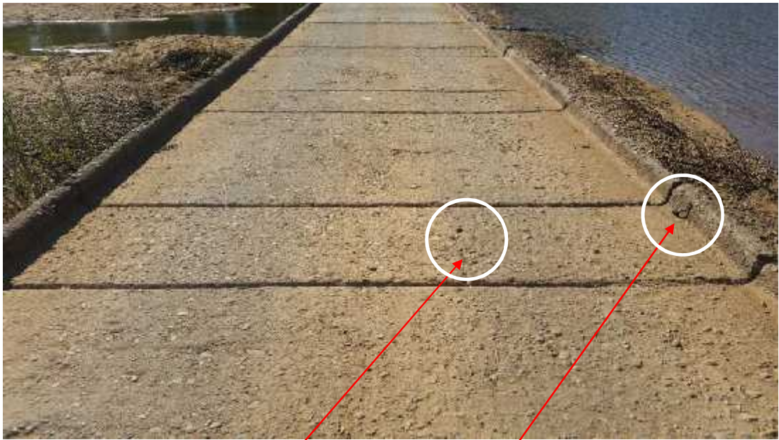
Longitudinal crack – 140023 – Reinforcing steel exposed
