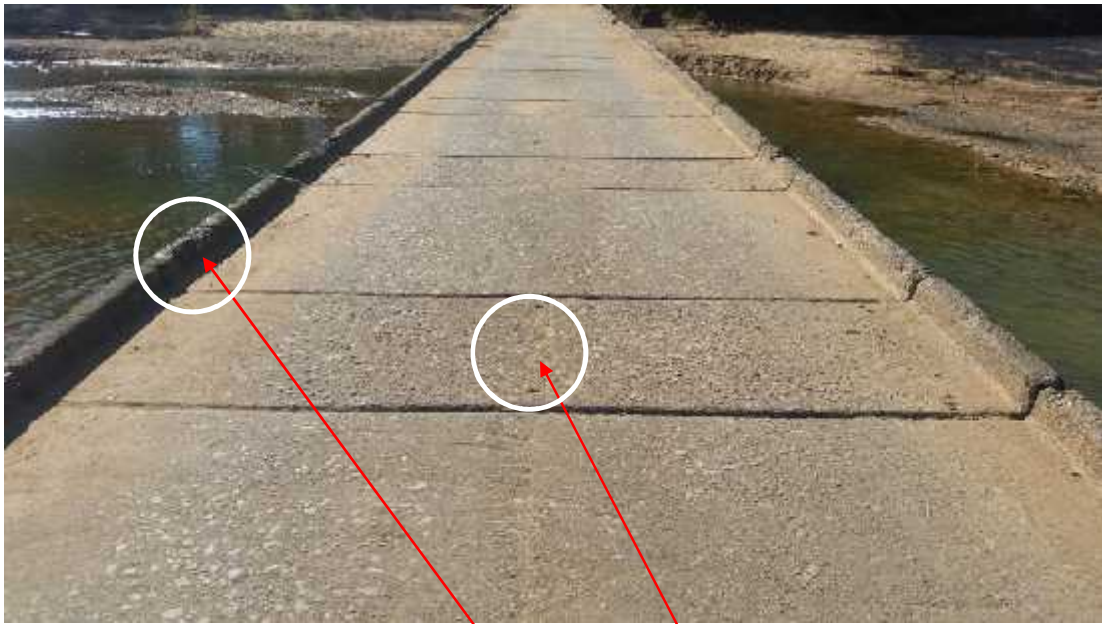
Spalling to kerb - 140246 – Longitudinal crack
