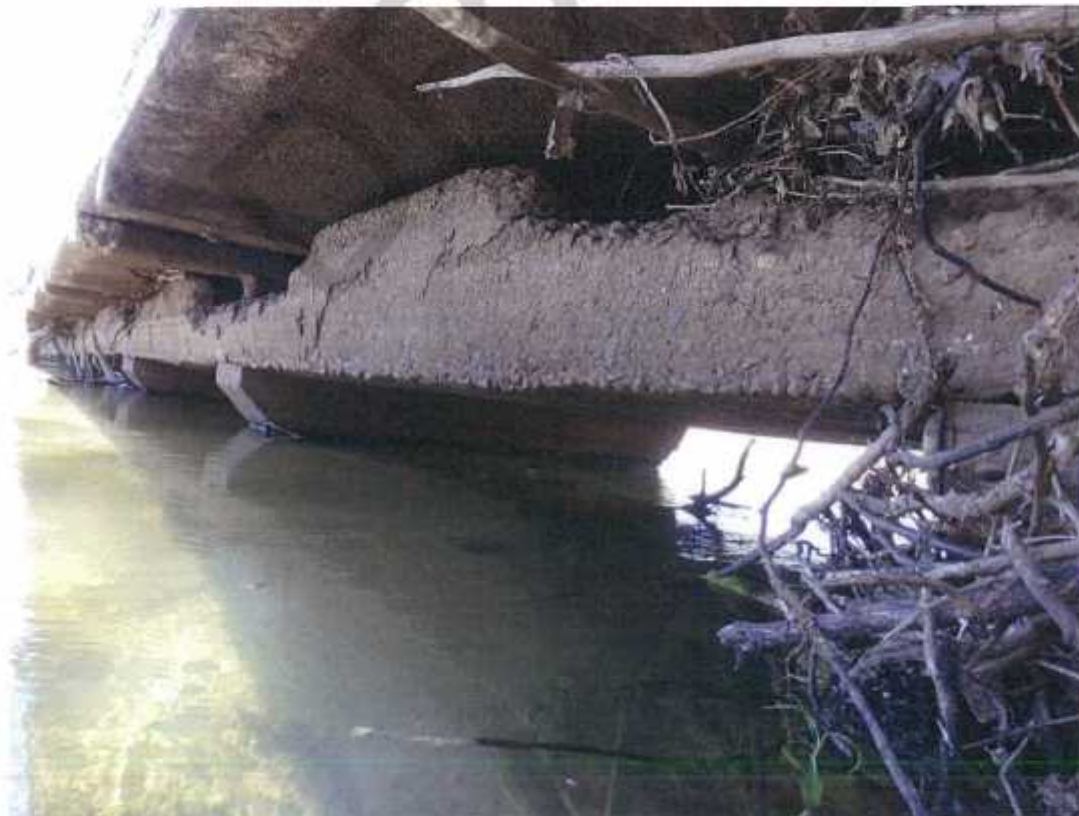
Photo No. 20: LHS span 10, cracking/ spalling to kerb edge. (Taken: 20-Jun-2016)
