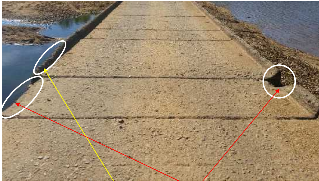
Kerb damaged – 135933 – Kerb missing
