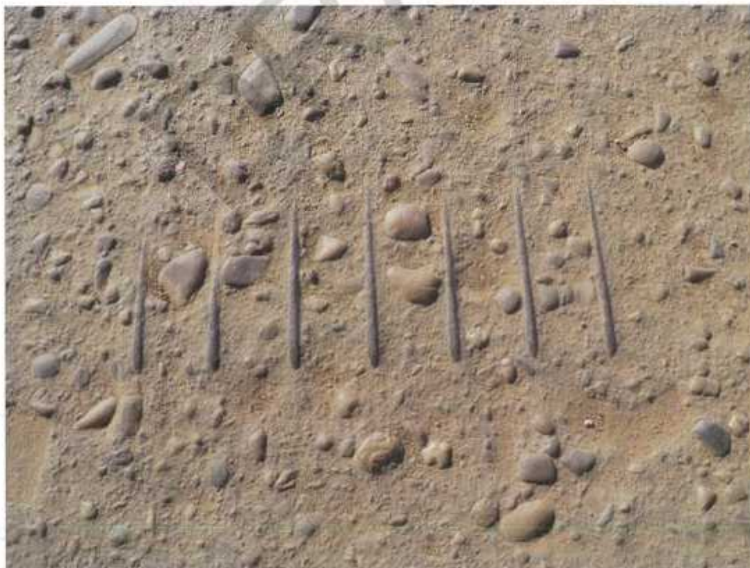
Photo No. 10: Typical area of poor cover to the reinforcement along the deck (Taken: 20-Jun-2016)
