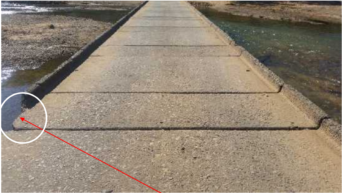
140223 – Part kerb missing
