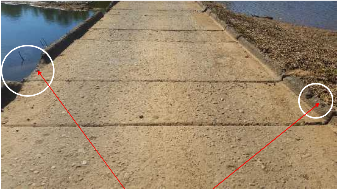
Part kerb missing – 135920 – Reinforcing steel exposed
