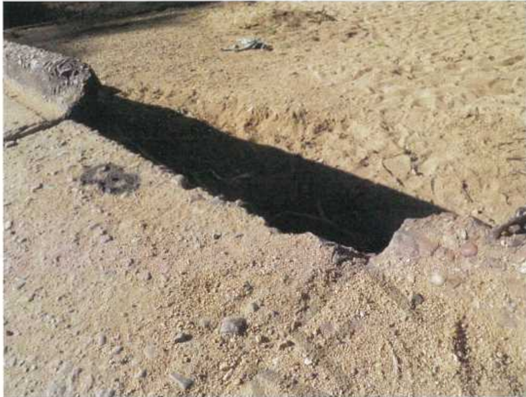
Photo No. 7: Typical broken kerb - LHS (Taken: 20-Jun-2016)
