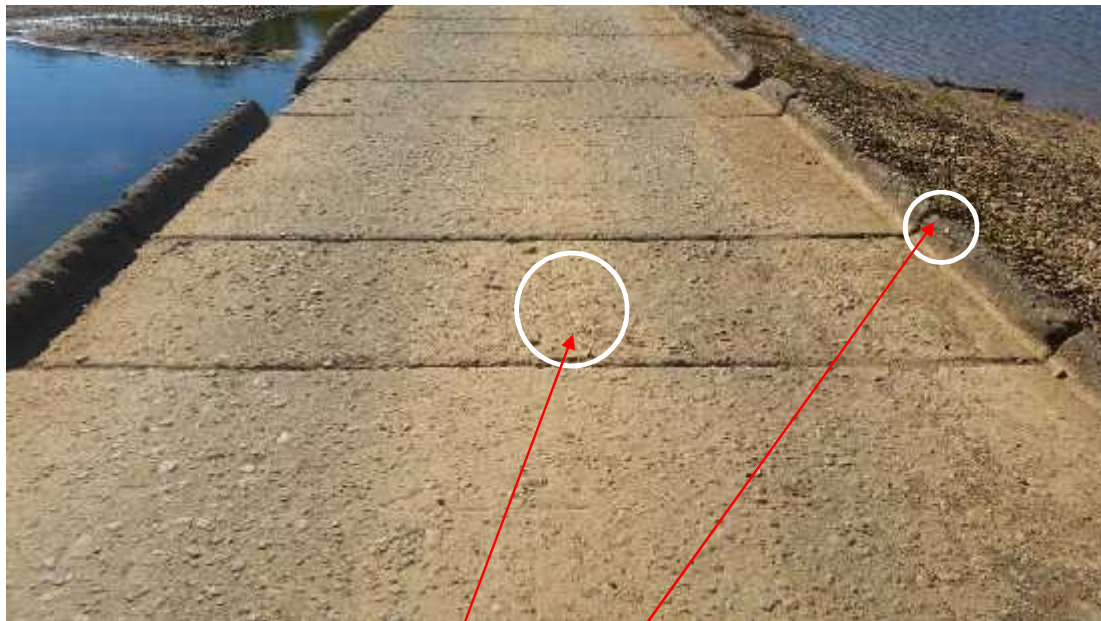
Longitudinal crack – 135926 – Reinforcing steel exposed
