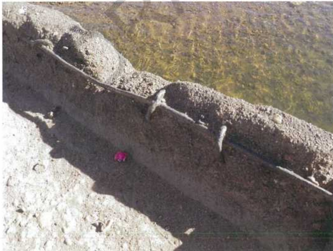
Photo No. 8: Typical spalling and exposed reinforcement - RHS kerb (Taken: 20-Jun-2016)
