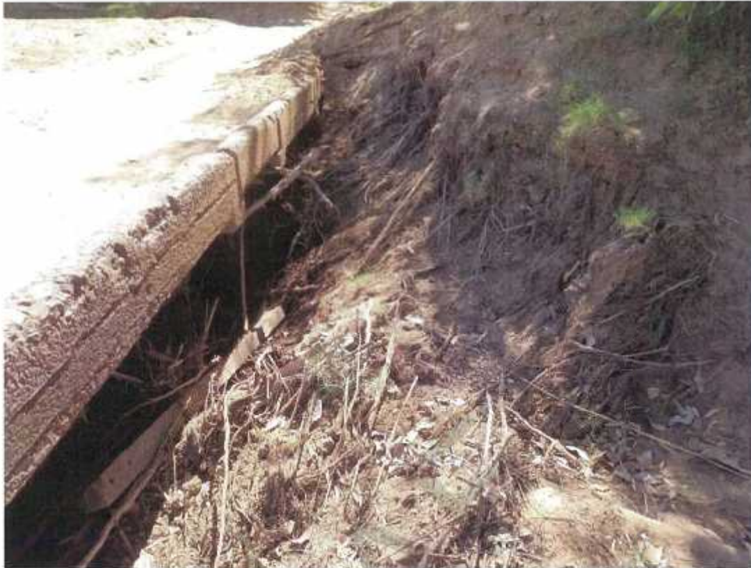
Photo No. 17: LHS span 5, wash-out to embankment, (Taken: 20-Jun-2016)
