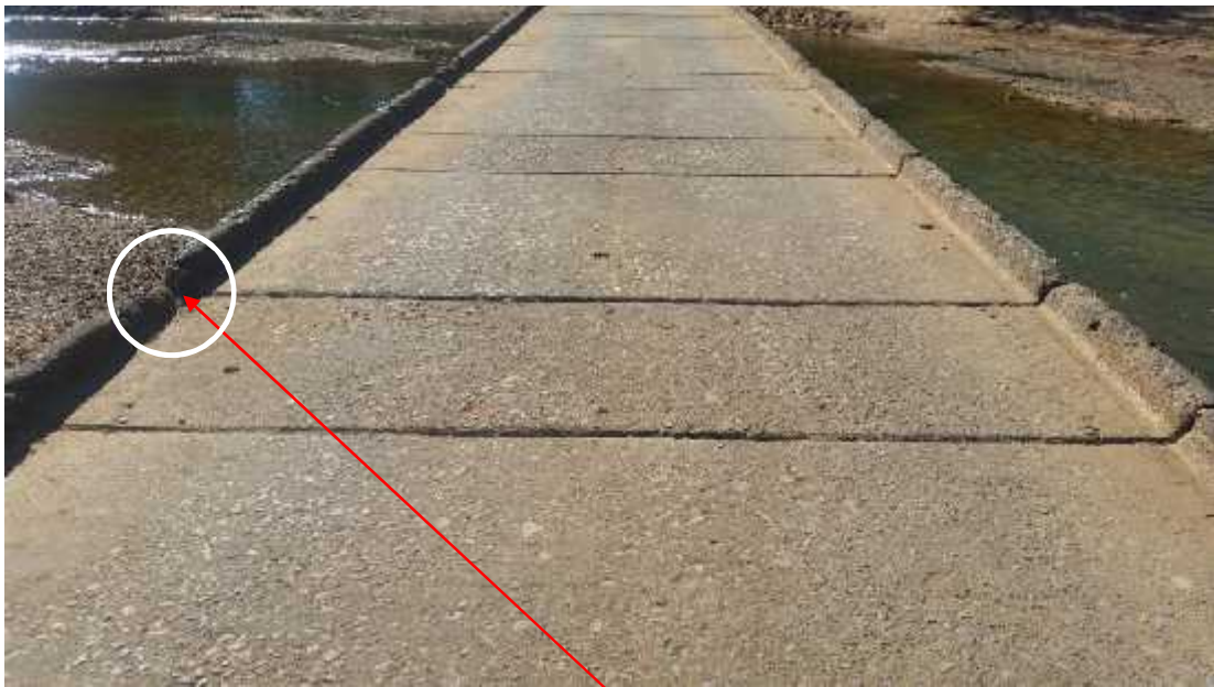
140240 – Kerb abraded and reinforcing steel exposed
