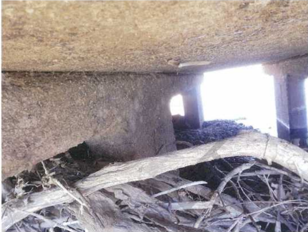
Photo No. 31: LHS at pier 30 (A2 side), legs to span 31. (Taken: 20-Jun-2016)
