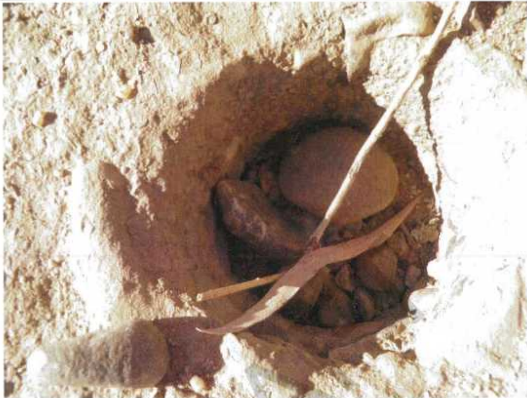
Photo No. 13: Typical blocked drainage hole (Taken: 20-Jun-2016)
