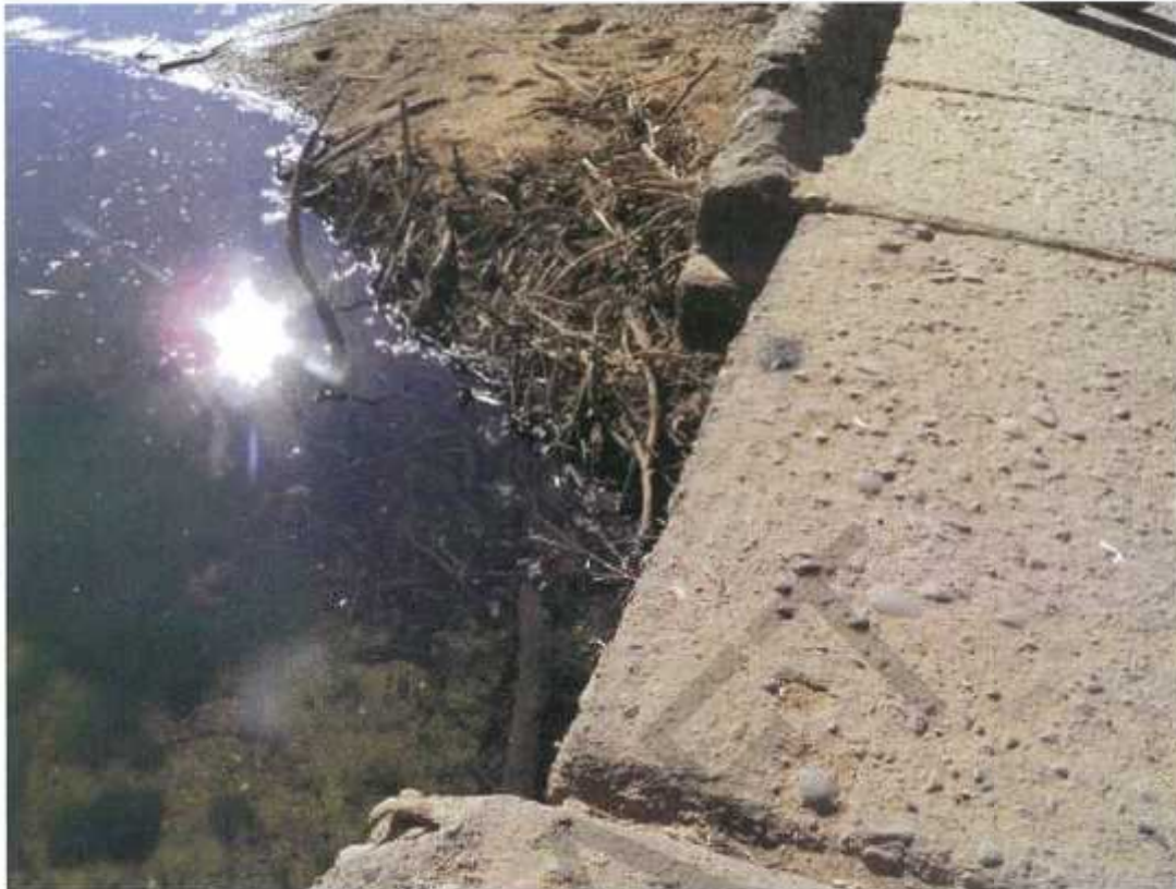
Photo No. 9: Typical broken kerb - RHS (Taken: 20-Jun-2016)
