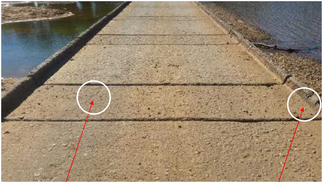
Longitudinal crack – 140035 –Reinforcing steel exposed
