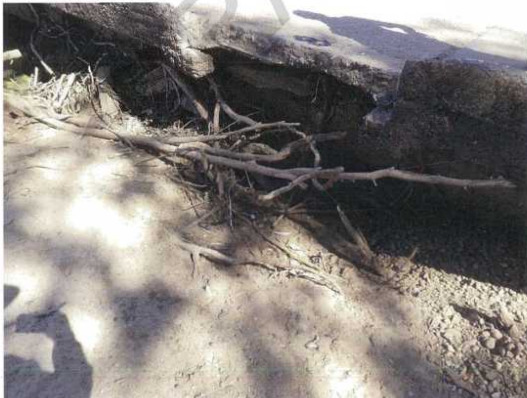
Photo No. 18: LHS pier 8, flood debris, (Taken: 20-Jun-2016)
