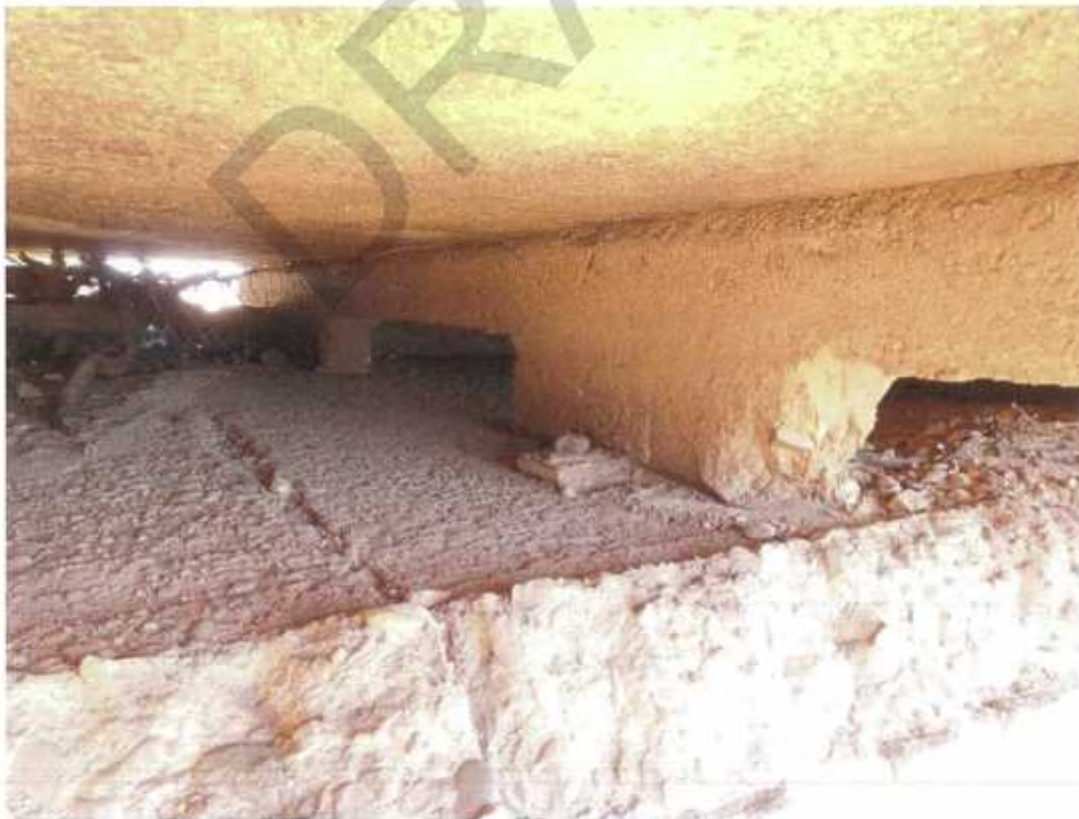
Photo No. 46: RHS at pier 8, A2 legs spalled. (Taken: 20-Jun-2016)
