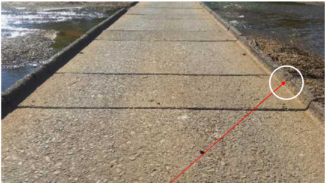
140206 – Reinforcing steel exposed
