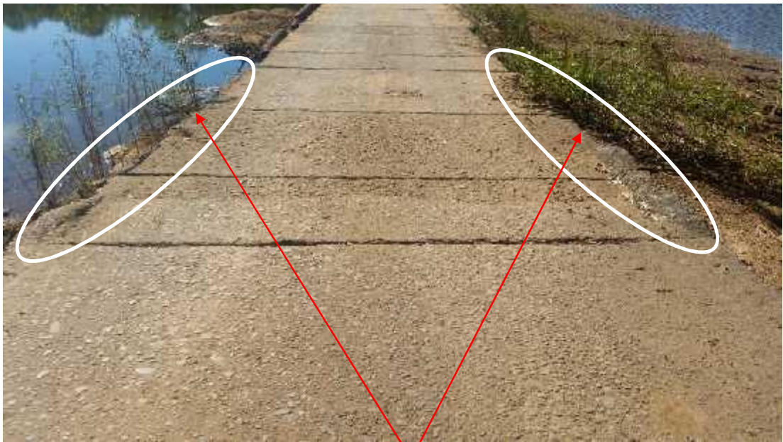
135818 Missing / abraded kerbs
