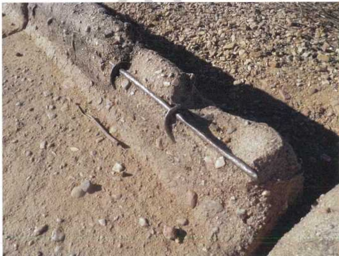
Photo No. 6: Typical spalling and exposed reinforcement - LHS kerb (Taken: 20-Jun-2016)
