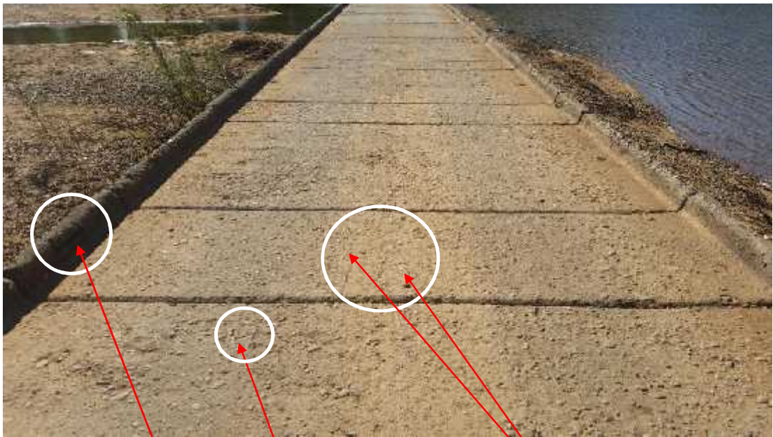
Spalling and reinforcing steel exposed – 140018 – Longitudinal cracks
