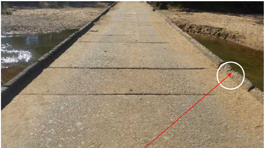
140306 – Reinforcing steel exposed
