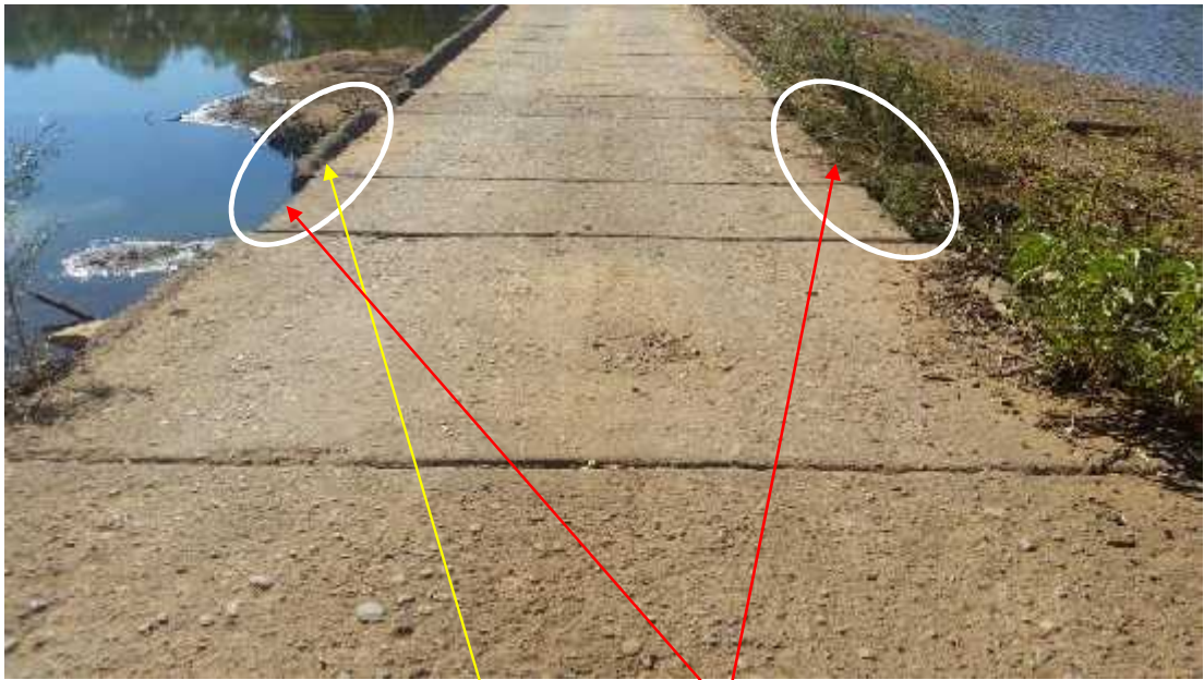
Abraded kerb – 135829 – Missing kerb
