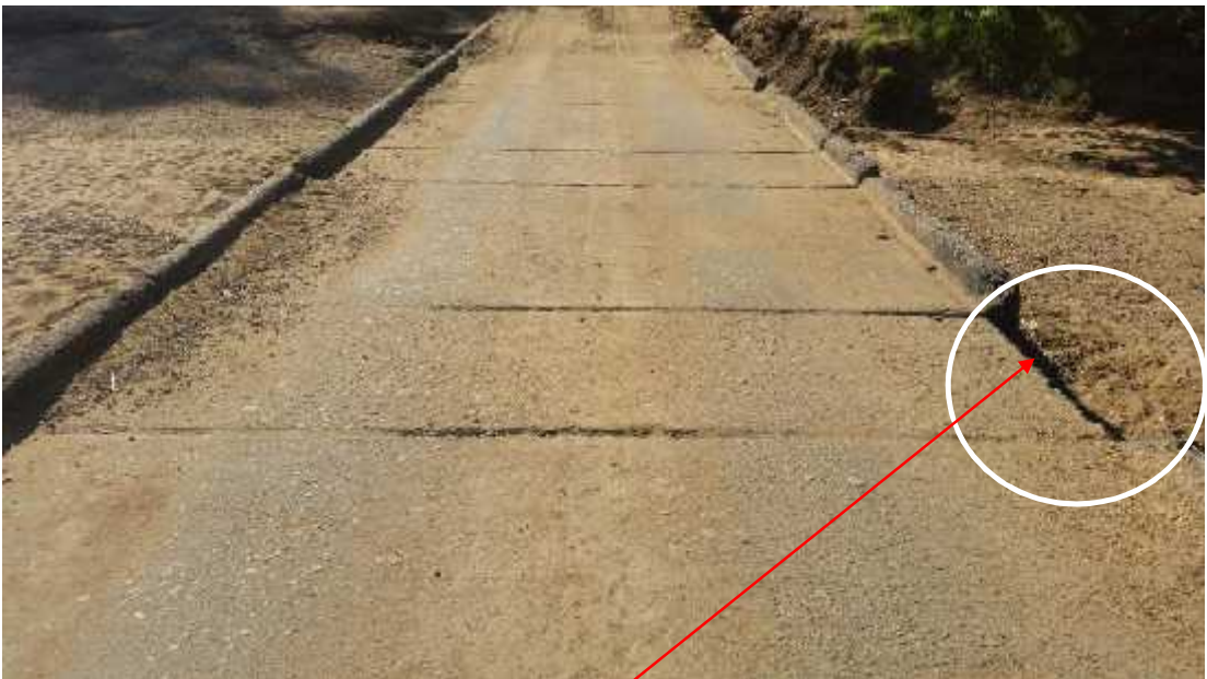
140330 – Kerb completely missing
