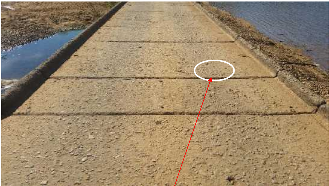
135941 - Reinforcing steel exposed
