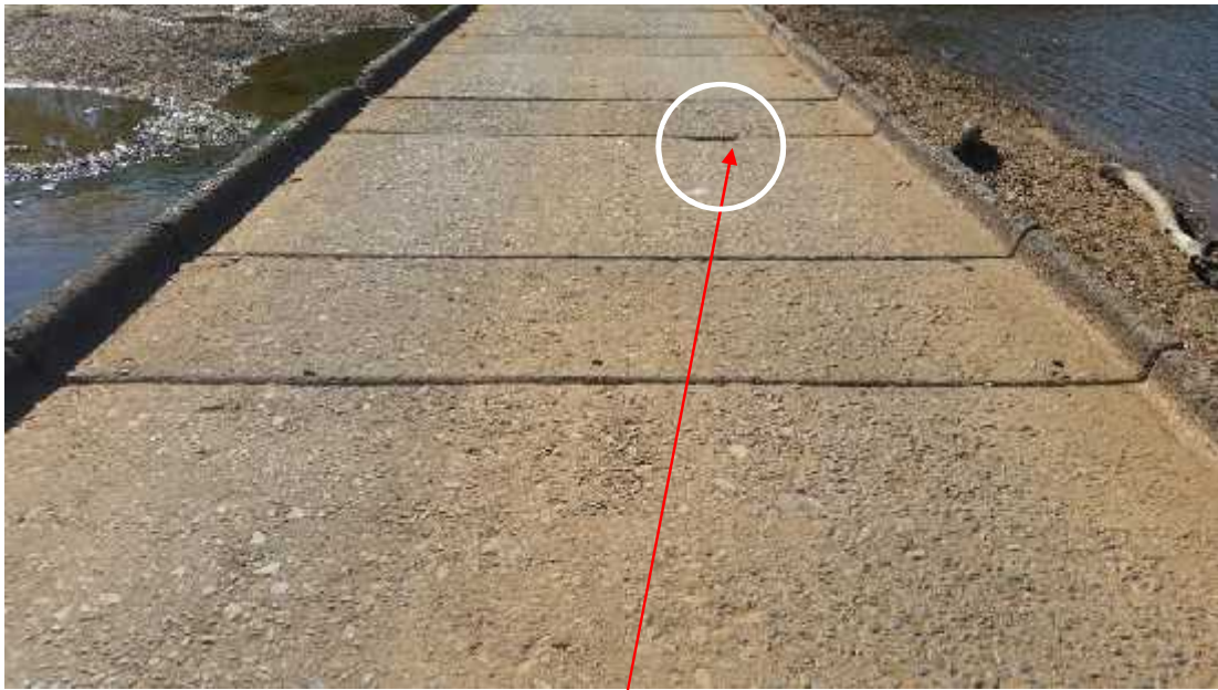
140127 – Spalling and reinforcing steel exposed (see 140154 above)
