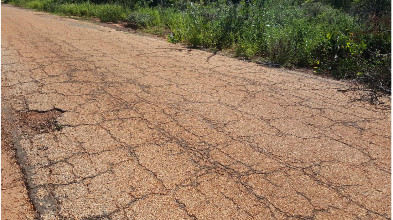
Crocodile Cracking, Granville St – Condition 5, Very Poor
