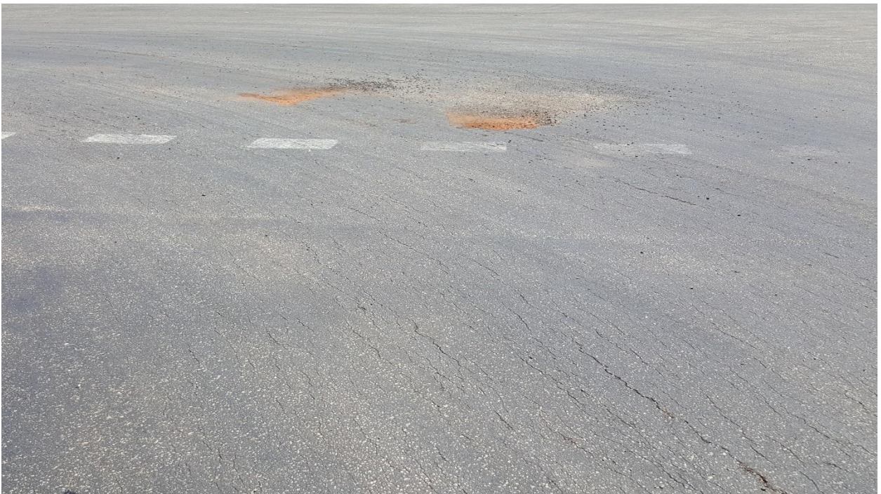
Deformation (shoving), Jetty Access Road – Condition 4, Poor
