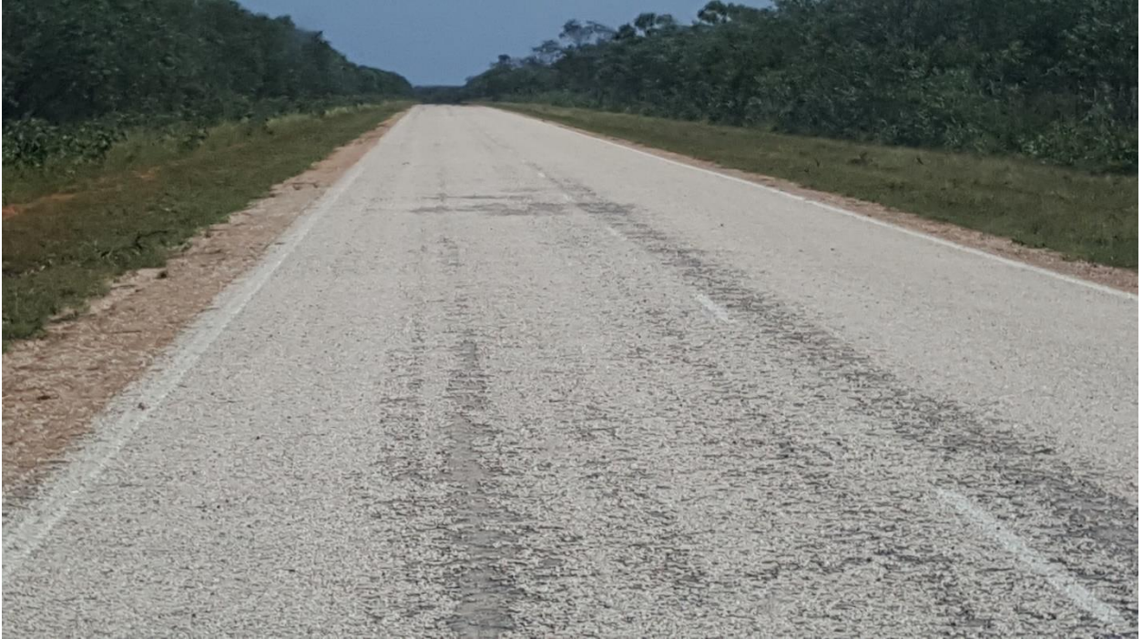
Ravelling (fretting), Curtin Access Rd – Condition 5, Very Poor
