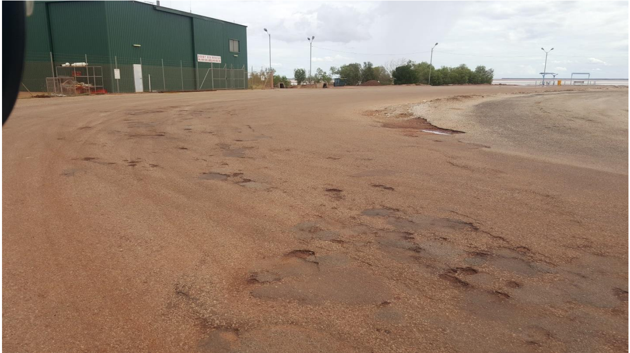
Potholing, Jetty Boat Ramp Access Road – Condition 5, Very Poor
