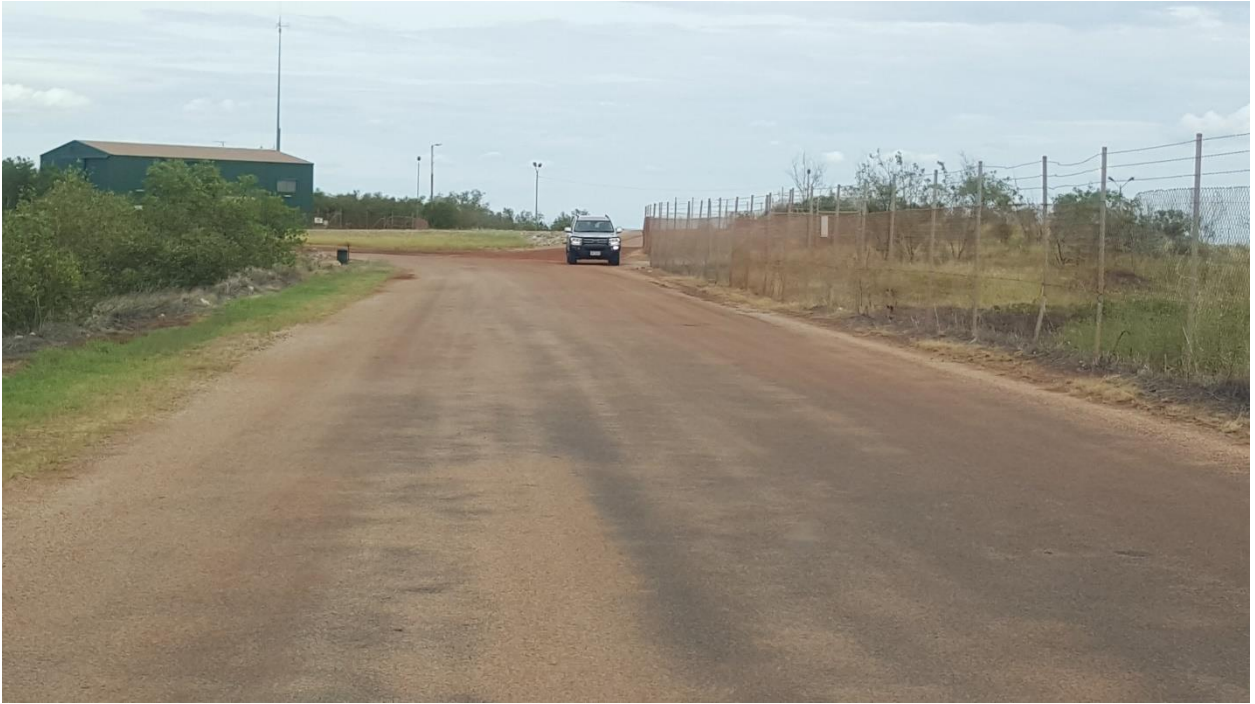
Flushing (bleeding), Jetty Boat Ramp Access Road – Condition 5, Very Poor
