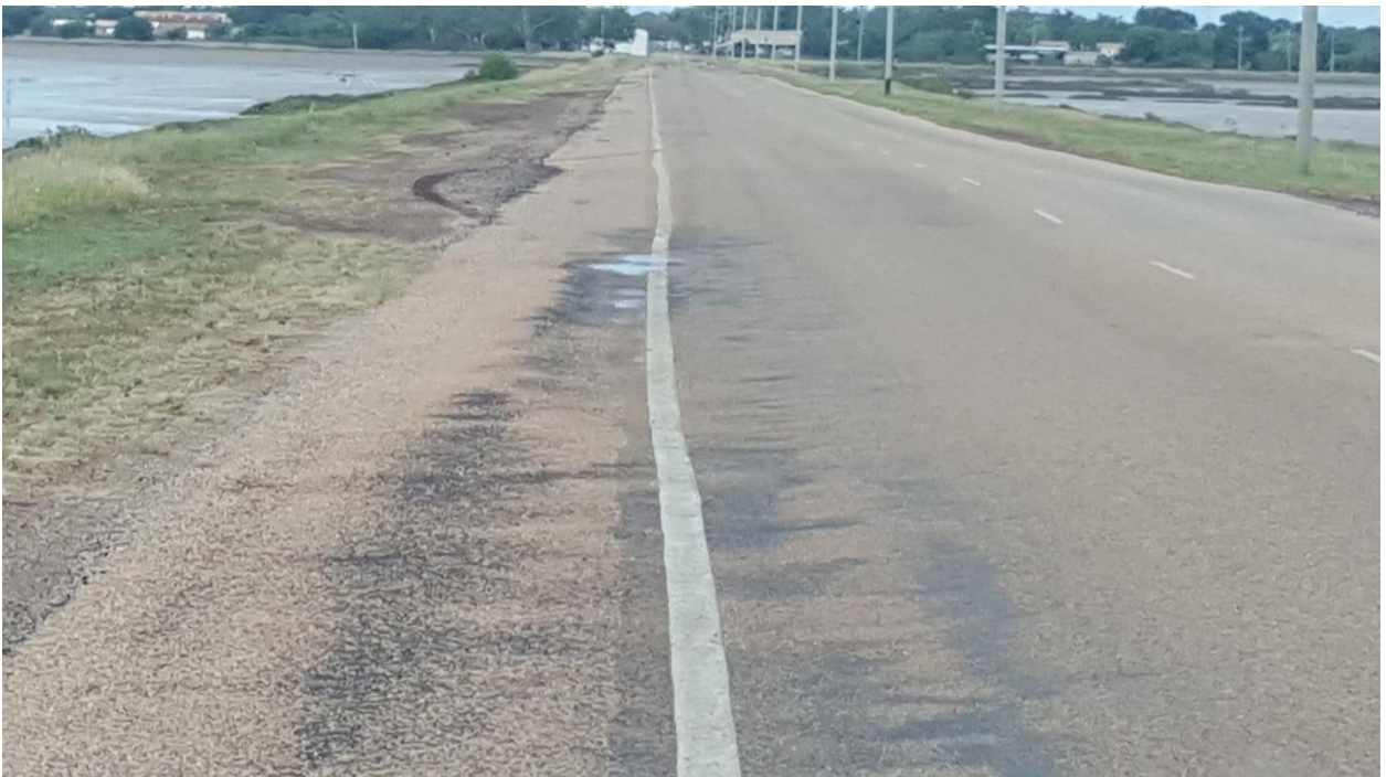
Deformation (rutting), Jetty Rd – Condition 4, Poor
