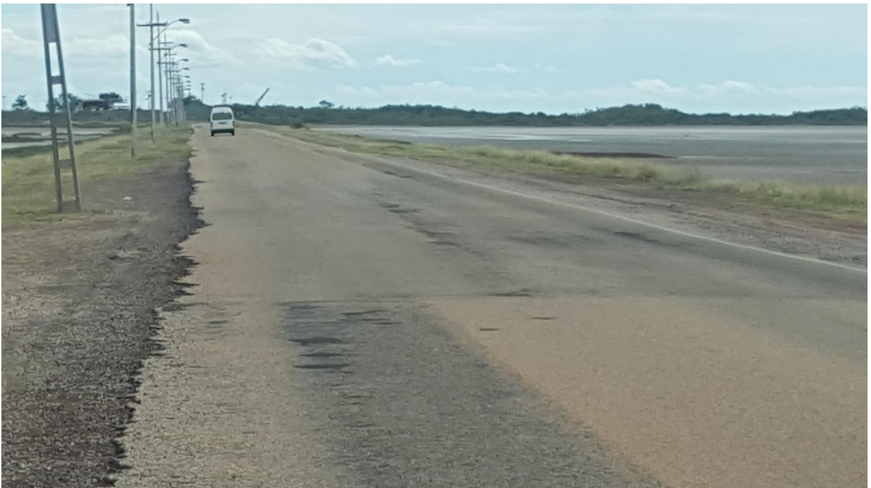
Edge Break, Jetty Rd – Condition 4, Poor
