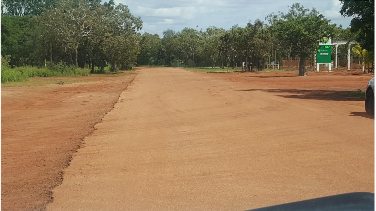
Edge Drop Off, Rodgers St – Condition 4, Poor
