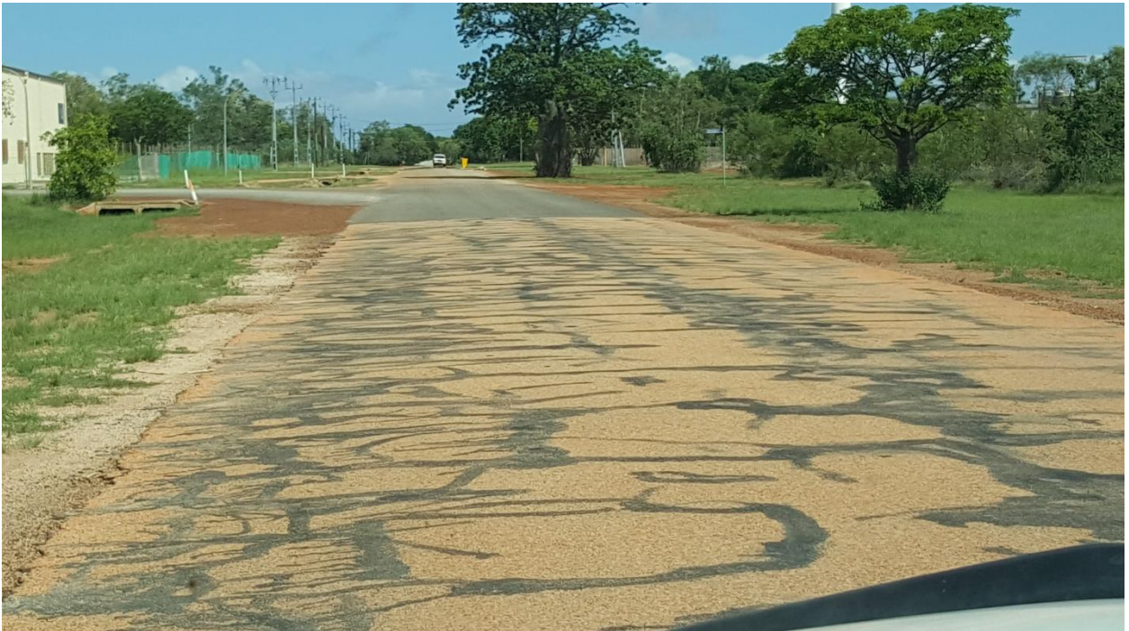
Transverse Cracking, Wodehouse St – Condition 5, Very Poor
