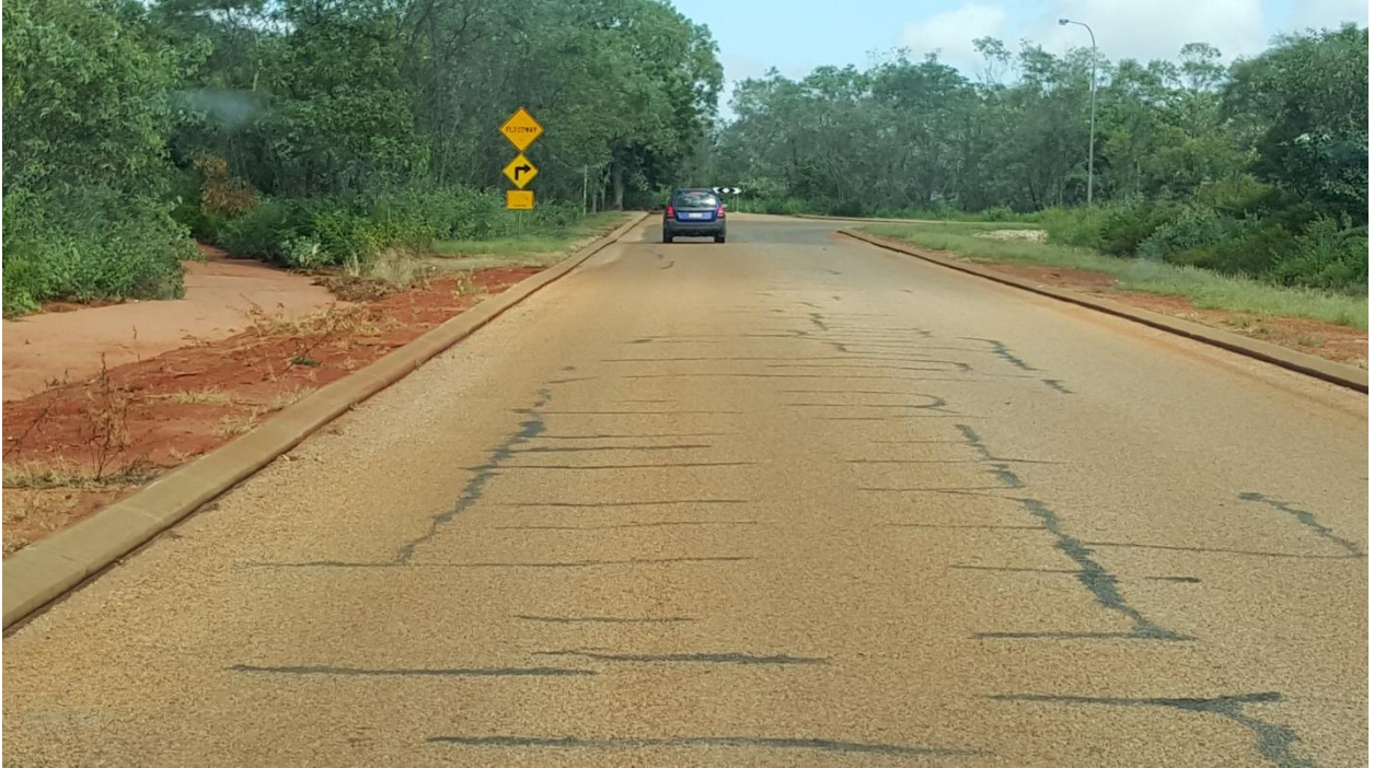
Block Cracking, Fitzroy St – Condition 3, Fair
