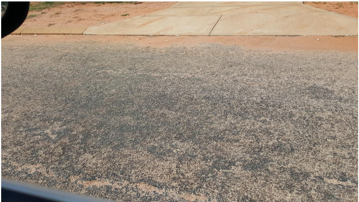
Polishing, Short St – Condition 5, Very Poor
