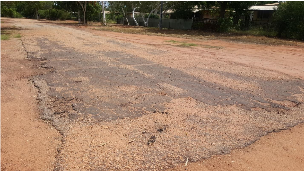
Stripping, Rowell Crt – Condition 5, Very Poor
